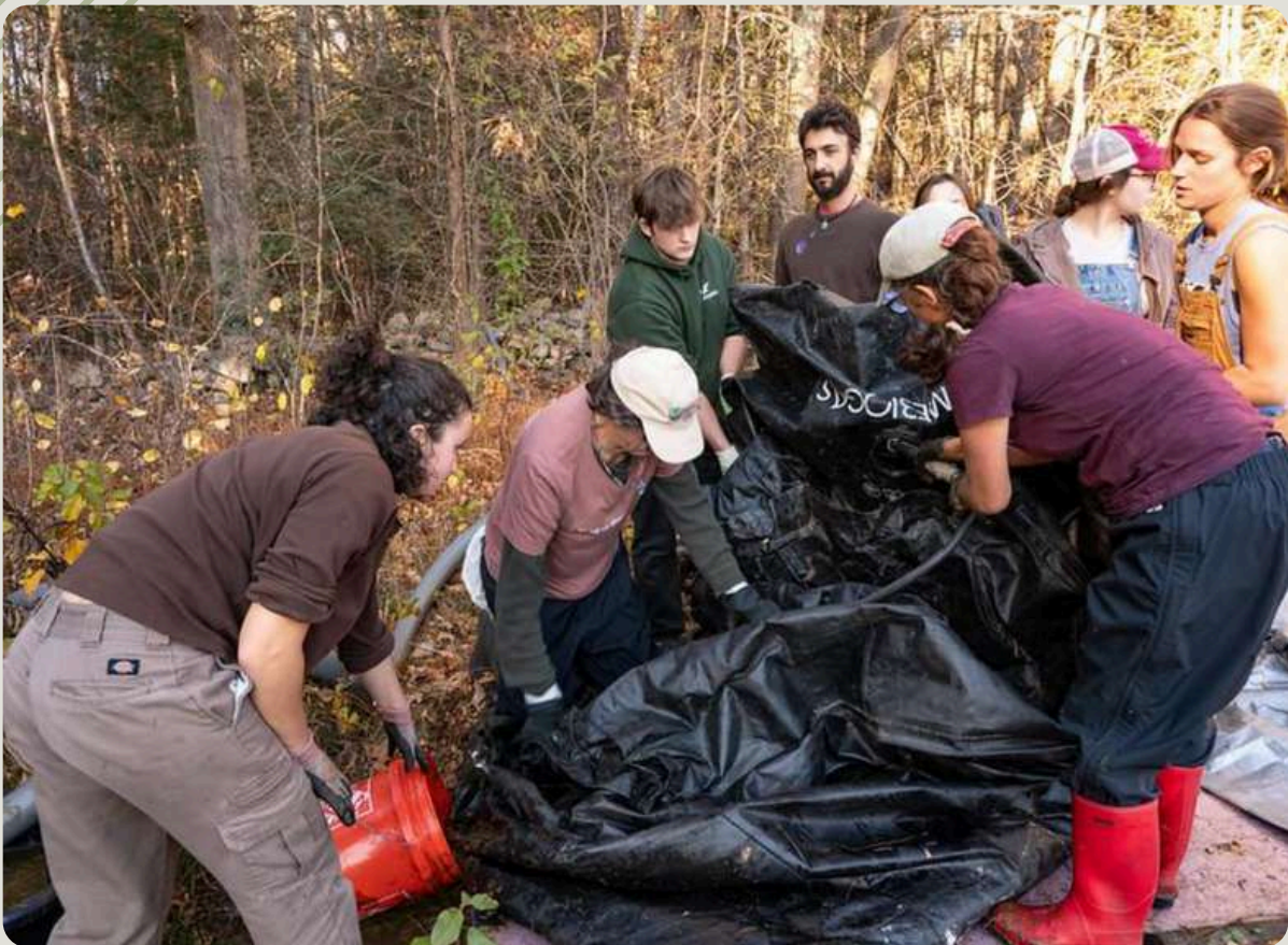
Working with the Northeast Biogas Initiative to install a biogas digester for the Franklin Garden
